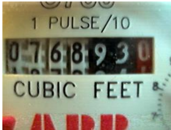
Figure 25 Original utility meter image #2
